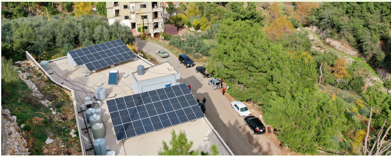
Figure 2. 25-kWp solar PV hybrid on-grid rooftop system, with a 90-kWh battery capacity in Akkar Al-Atika serving Union of Beekeepers Cooperative building, municipality building, and clinic
