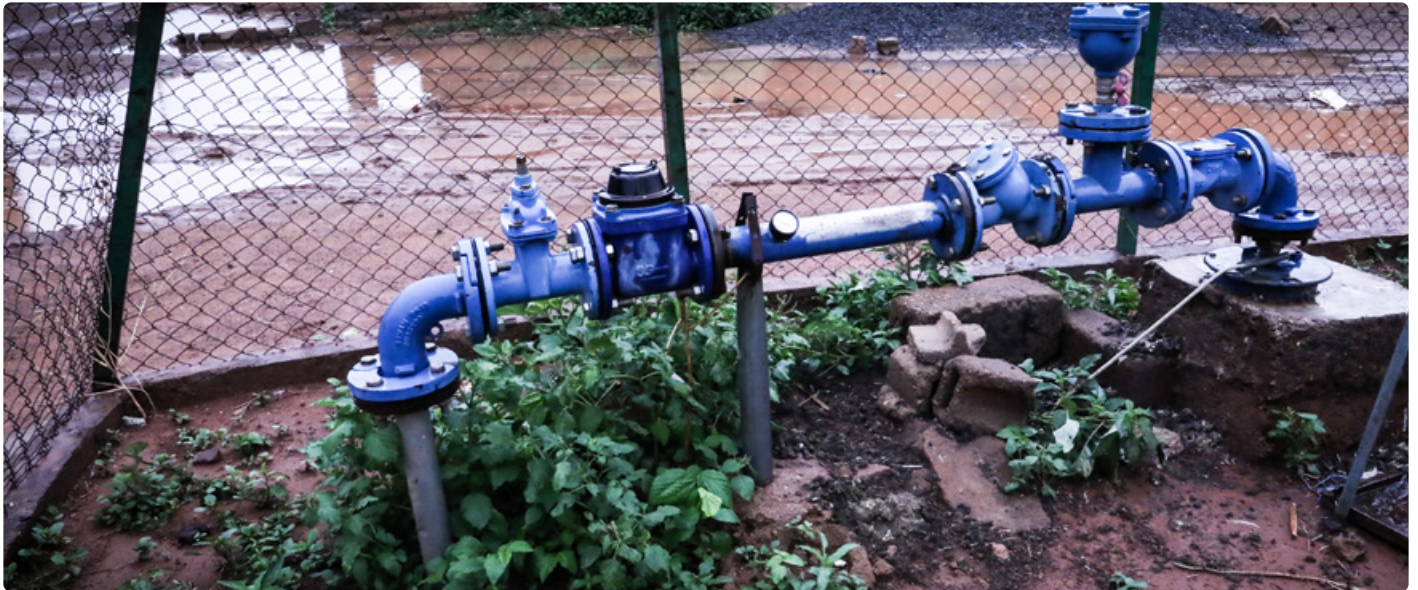
Dialakorodji's solar-powered pump. ©UNDP
